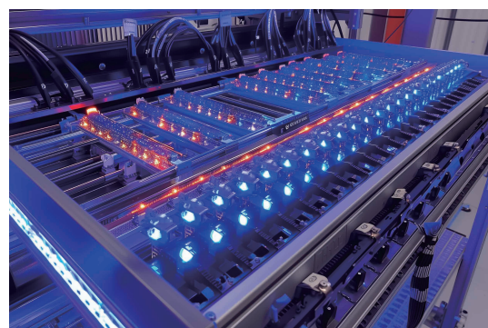
Liquid cooled data center
